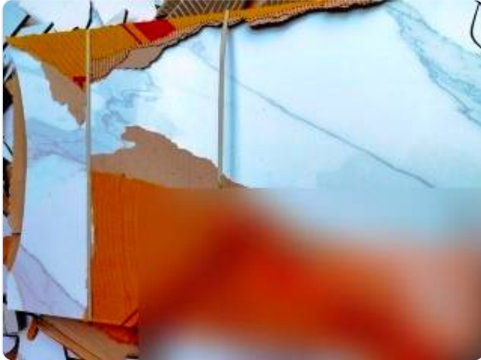
Photo 1: Fractured large-format tiles with crushed cardboard packing | Geotag overlay redacted
